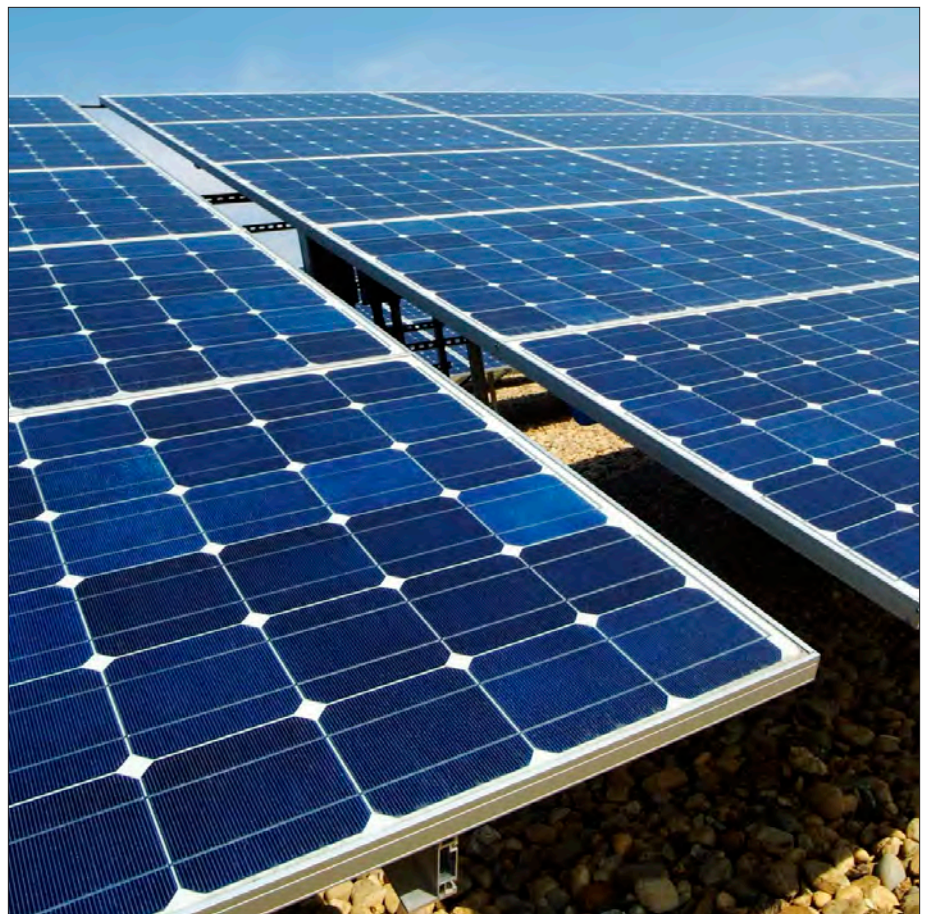
On-site Power Generation
